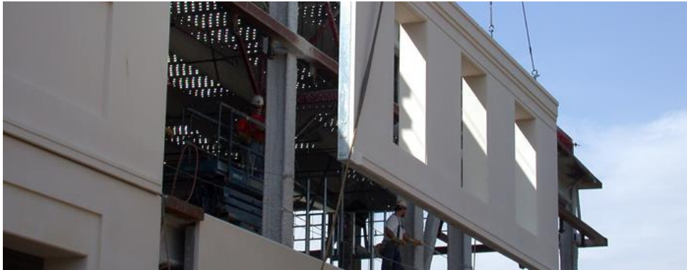
Façade Cladding Panels
